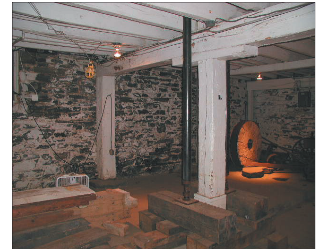
The jacks in position at Column #1 at the basement level, preparatory to removal for inspection. Also visible is the column at the south wall, which will be the next to be examined.
