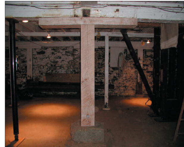
The completed work on Column #2, showing the new post and capital in place.
