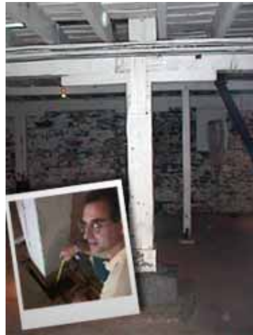
Rocky Footing. The column supporting the second floor has migrated eastward (toward the camera) due to a large crack in the horizontal beam. Note the vertical alignment with the lower column is off center. Inset: Steve Ortado measures the depth to which the post has sunk into the rotting main beam.
