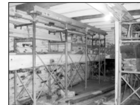
Scaffolding erected in basement to support the millstone load on the main floor.
