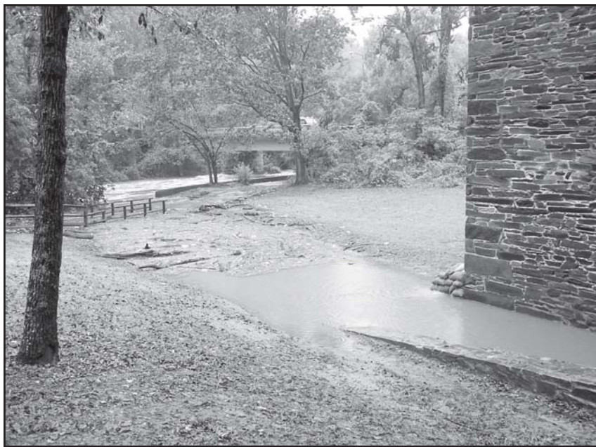
This shows what Rock Creek can do to the mill after a heavy rain. Photo taken on October 8, 2005.
